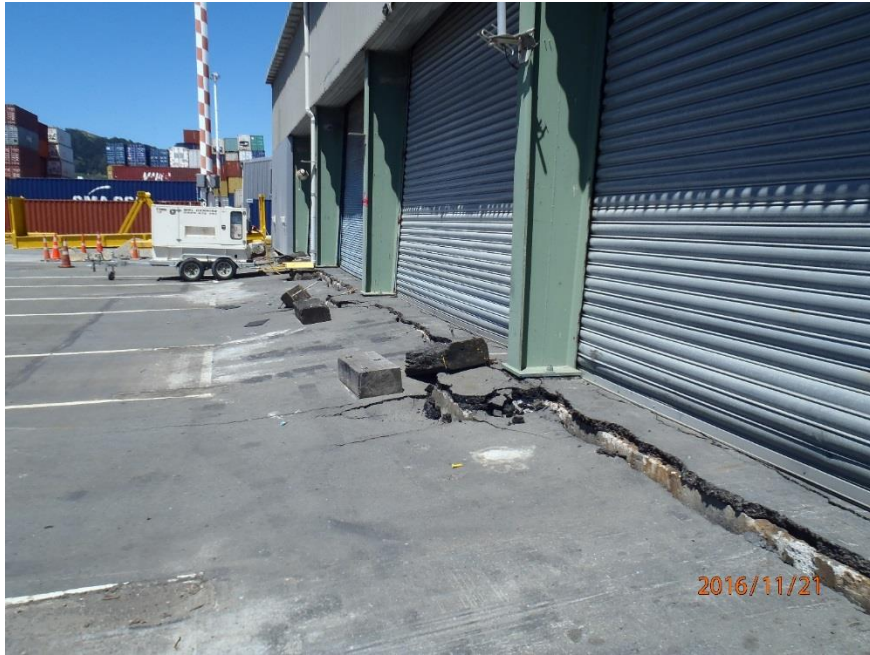
Figure 5.76: Looking south along east wall of Building S37, which shows approximately 375 mm of differential settlement between fill and pile-supported east wall of the building. (S41.279065°, E174.785787°, taken at 1220 hrs on 21NOV16)
