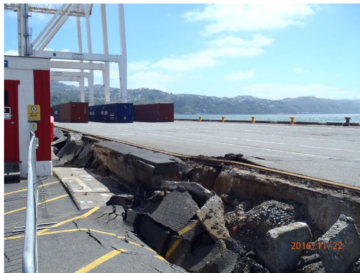
Figure 5.36: Looking north along Thorndon Wharf bulkhead at approximately STA 280. Approximately 600 mm of ground settlement measured relative to pile-supported wharf. (S41.277743° E174.789236°, taken on 22NOV16)
