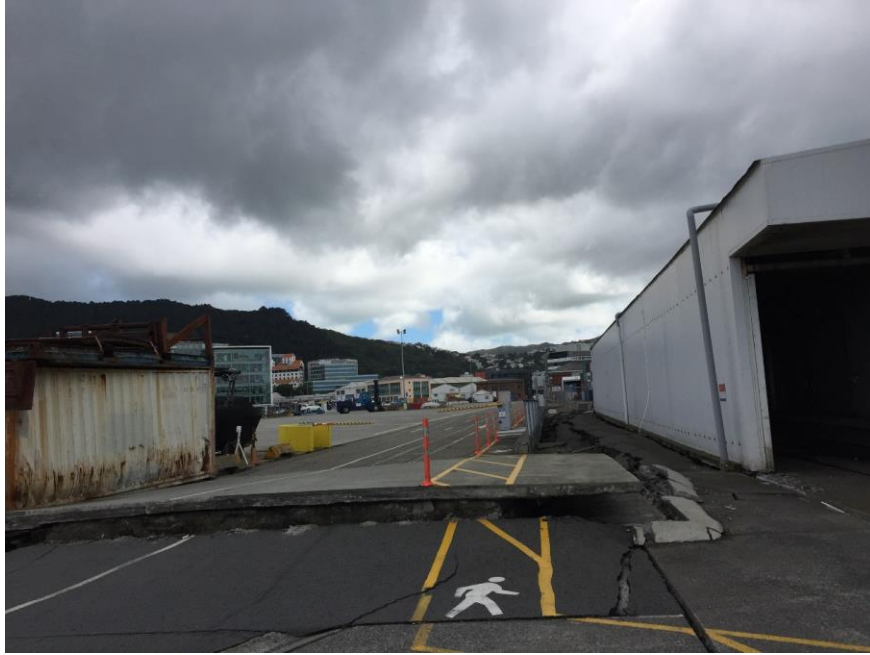
Figure 5.42: Looking North along bulkhead of King's Wharf. Approximately 560 mm of ground settlement relative to deck at southeast corner of King's Wharf. The west wall of the Cold Store shed is visible to the right of the photograph. (S41.281142° W174.784444°, taken at 1416 hrs on 21NOV16)
