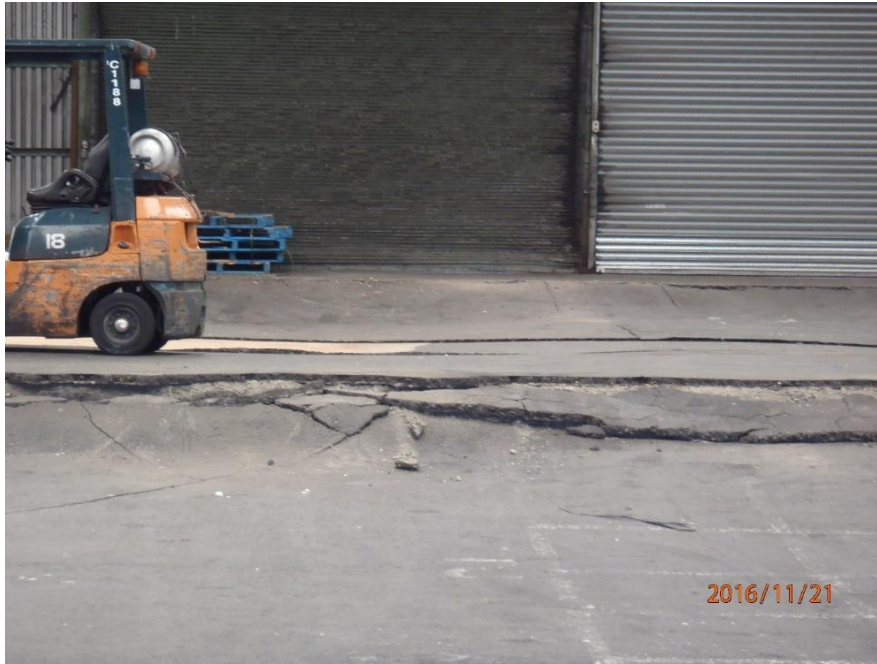
Figure 5.72: Looking west across inside of the S37 building. Approximately 400-550 mm of differential settlement between the ground and the buried precast concrete seawall that runs south-to-north through the center of the building. (S41.279065°, E174.785787°, taken at 1220 hrs on 21NOV16)
