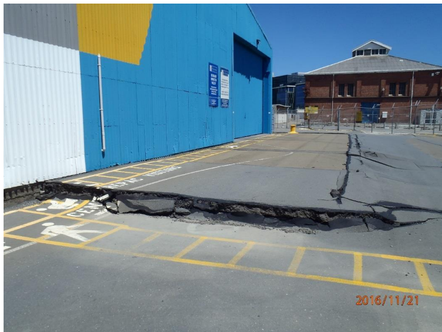
Figure 5.73: Looking west across north wall of Building S37. Approximately 400mm of differential settlement between ground and deck of buried, pile-supported Pipitea Wharf that supports the western side of the shed. (S41.278571°, E174.785632°, taken at 1227 hrs on 21NOV16)
