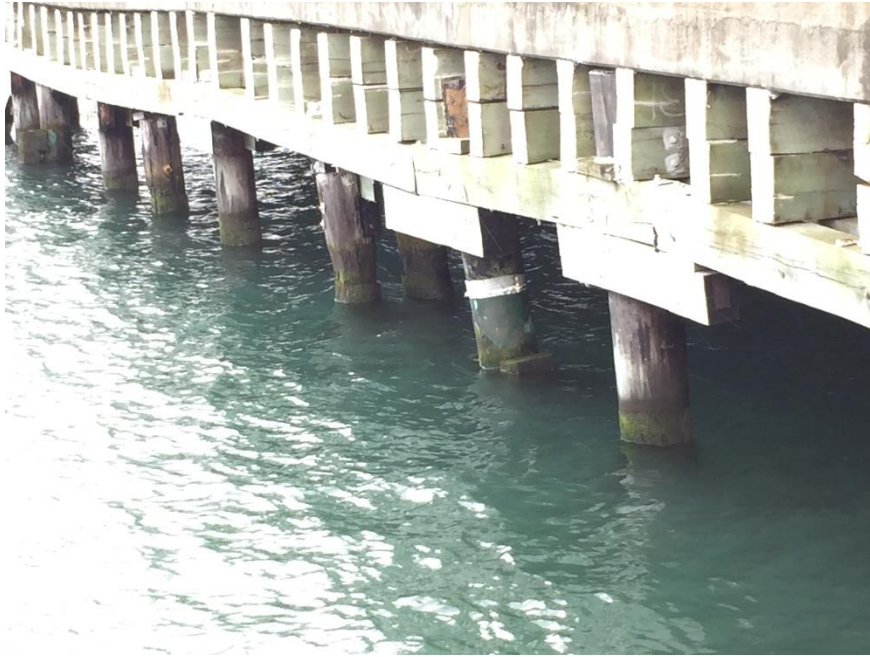
Figure 5.44: Looking west along southern end of King’s Wharf. Westward tilt of piles is visible. (S41.281281° W174.784097°, taken on 17NOV16)
