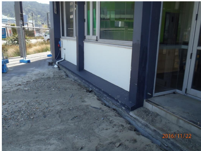
Figure 5.71: Southwest wall of TC building with liquefaction ejecta and 150 mm of ground settlement relative to building. (S41.277858°, E174.785081°, taken at 1246 hrs on 22NOV16)
