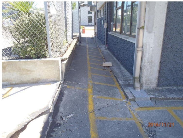
Figure 5.49: Uniform settlement (230-260 mm) of the building relative to ground supported on old bulkhead piles of Pipitea Wharf. Looking north along western wall of CPH building. The perimeter walkway slopes down towards the building at 11 degrees over 1.35 meters. (S41.278395° E174.785639°, taken at 1225 hrs on 22NOV16)
