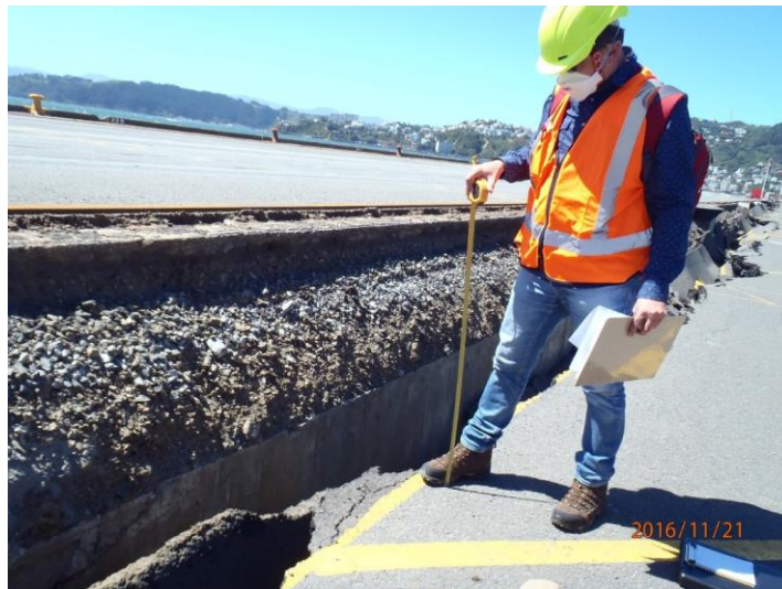
Figure 5.35: Looking south along Thorndon Wharf bulkhead at approximately STA 240. Approximately 600 mm of ground settlement measured relative to pile-supported wharf. (S41.278250° E174.789205°, taken at 1124 hrs on 21NOV16)
