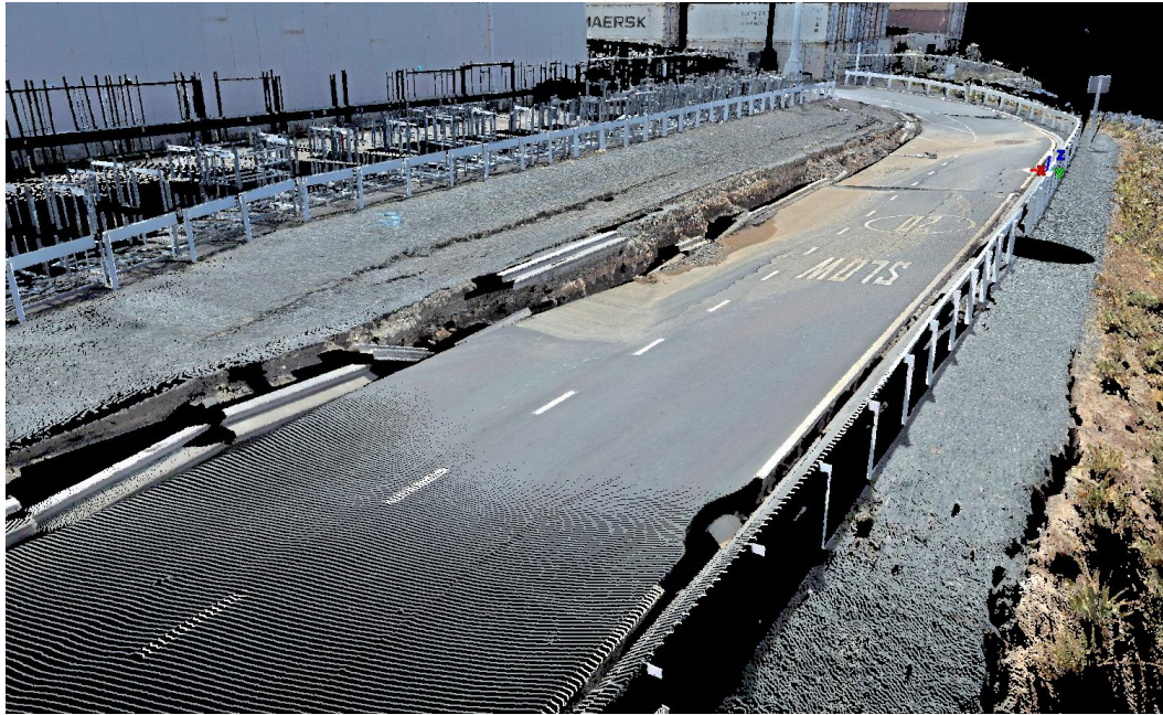
Figure 5.57: LiDAR scan of damage to the asphalt pavement and concrete curbs on the access road located south of the CS building. The vertical offset is approximately 1.1 m. This view is looking to the northeast.
