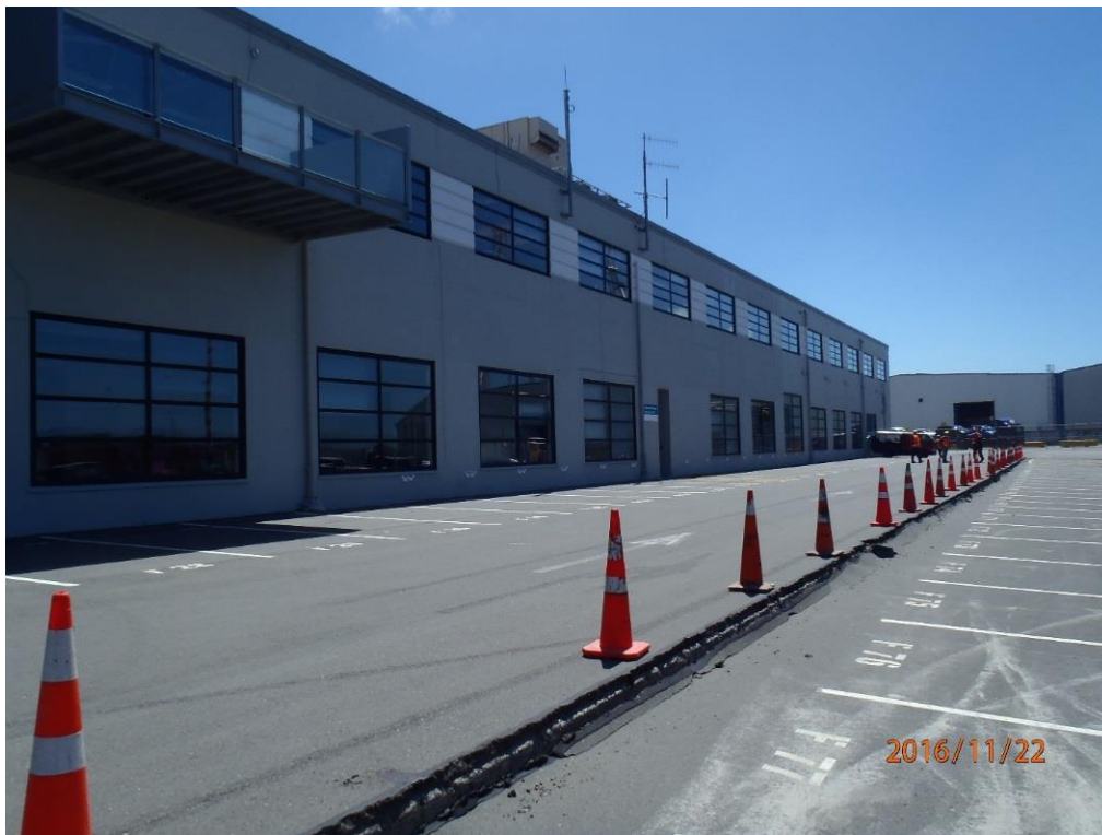
Figure 5.68: Southeast side of Building S39 and a buried segment of the Fryatt Quay Wharf deck parallel to the building. Fill to the south of the buried mass concrete seawall/wharf settled 220 mm relative to the pile-supported building and wharf deck. (S41.277984°, E174.785776°, taken at 1230 hrs on 22NOV16)
