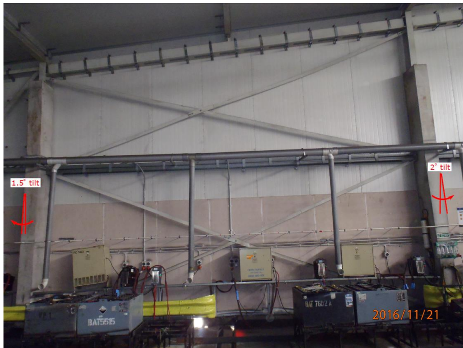
Figure 5.65: Internal north wall of Shed of CS building showing 1.5° clockwise tilt of the left column (2 nd column from the west along north wall), and 2° counterclockwise tilt of the right column (3 rd column from the west along north wall). This deformation was caused by a 180 mm opening in the RC base wall, which is visible in the bottom middle of the photograph where light is entering building. This column span is 8.789 m from centerline of column to centerline at a height of 1.5 m above the floor slab. (S41.280626° W174.784450°, taken at 1452 hrs on 21NOV16)
