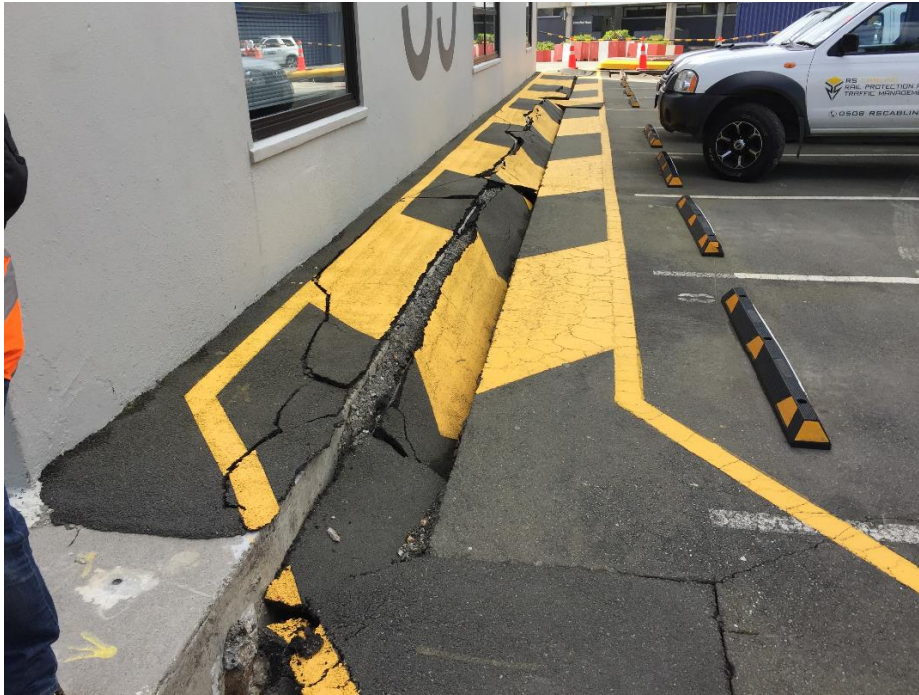
Figure 5.69: Looking southeast along southwest wall of S39. Fill settled approximately 190 mm relative to pile-supported building at the northwest corner of the building (shown on lower left corner of photo), and magnitude of settlement decreased south-eastward along this wall. (S41.277994°, E174.785467°, taken on 17NOV16)
