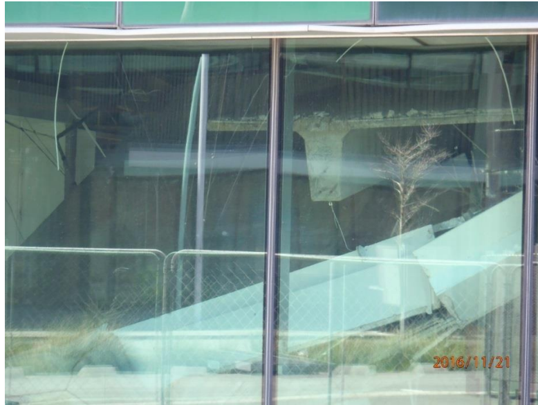
Figure 5.82: Pull-out and partial collapse of Level 1 floor slab in the S building taken along the west wall of the building. (S41.277982°, E174.784255°, taken at 1246 hrs on 21NOV16)
