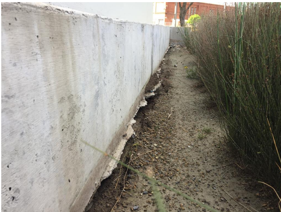
Figure 5.70: Looking southwest along northwest wall of S39. Fill settled 50-100 mm relative to pile-supported building. (S41.277882°, E174.785371°, taken on 17NOV16)
