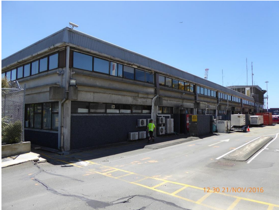
Figure 5.48: Uniform settlement of CPH building which is founded on shallow foundations that apparently displaced downward the same amount as the surrounding fill. This photo is looking northeast at the southwest corner of the building. (S41.278395° E174.785639°, taken at 1230 hrs on 21NOV16)
