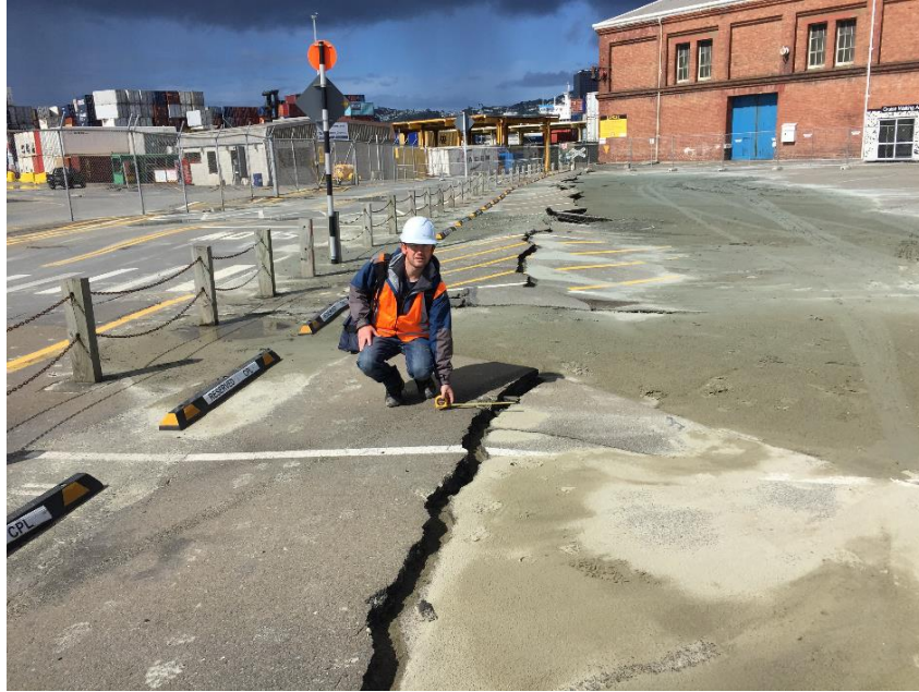
Figure 5.20: Sandy liquefaction ejecta behind buried mass concrete seawall looking southwest along seawall. On the right side of seawall: area of end-dumped quarry rock reclamation from 1904-1916 (Sample S2), left side of seawall: area of end-dumped quarry rock reclamation from 1970's Thorndon Reclamation. (S41.278454°, E174.785154°, taken on 17NOV16)
