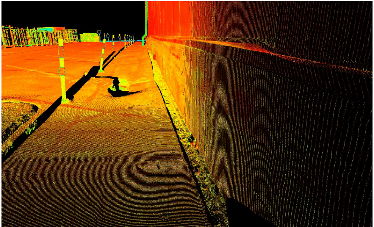
Figure 5.52: Perspective view of LiDAR scan looking westward showing the horizontal separation from building foundation and settlement of pavement observed on the south side of the CS building looking west (colored indicates intensity). The separation varies from 0.23 m wide to 0.03 m wide horizontally from the building's eastern side to its western side.
