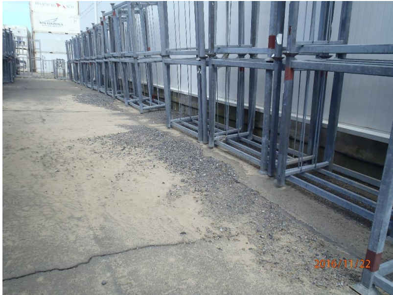
Figure 5.53: Gravelly liquefaction ejecta looking east along the northern wall of the CS building. (S41.280528° E174.784984°, taken at 1651 hrs on 22NOV16)
