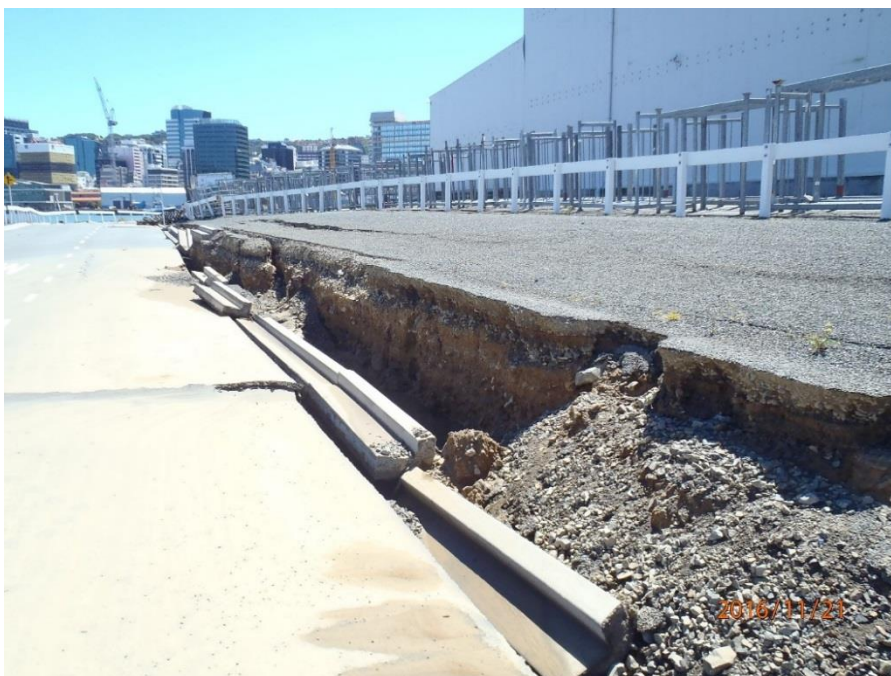
Figure 5.56: Approximately 1.1 m of vertical offset resulting from the southward lateral movement of the southern edge of CentrePort reclaimed land near its western side. Looking west near the southern wall of the CS building. (S41.281701° E174.785268°, taken at 1427 hrs on 21NOV16)
