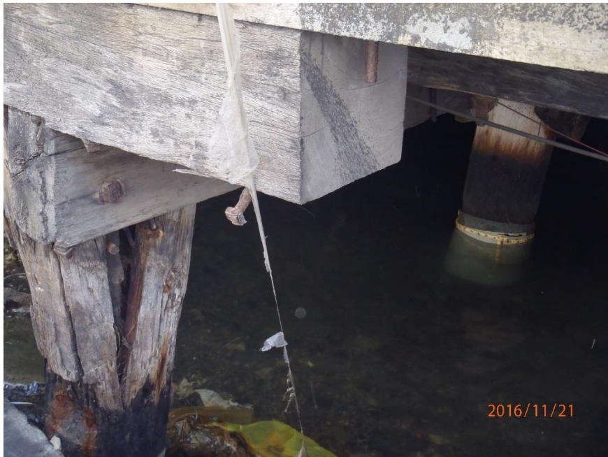
Figure 5.43: Looking under King's Wharf at an inland bulkhead pile. Timber pile is split from lateral movement (seaward/westward) of the deck relative to the pile. (S41.280900° E174.784375°, taken at 1412 hrs on 21NOV16)
