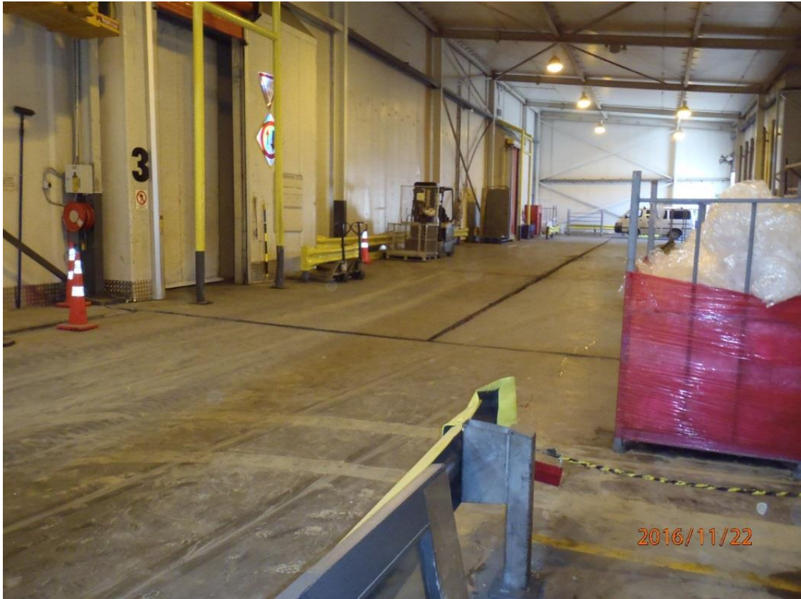
Figure 5.63: Contraction joint separation of ground floor slab inside the Shed of CS building looking south. As shown in photo, joint separations occurred in two orthogonal directions. (S41.281255° E174.784797°, taken at 1520 hrs on 22NOV16)
