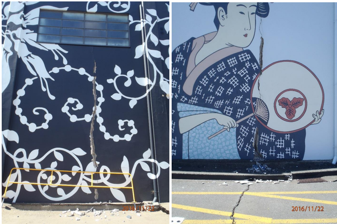
Figure 5.79: Vertical cracks along exterior west wall of S51 located at approximately 25 meters (left photo), and 60 meters (right photo) north of the southwest building corner. (Left: S41.272224°, E174.787391°, taken at 1316 hrs on 22NOV16. Right: S41.271906°, E174.787307°, taken at 1312 hrs on 22NOV16)
