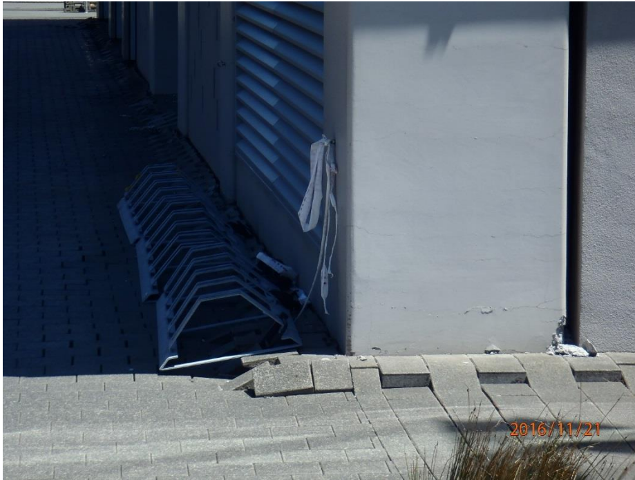
Figure 5.80: Looking west at southeast corner of the S building at which fill settled approximately 100 to 200 mm relative to pile-supported building. (S41.278285°, E174.784757°, taken at 1243 hrs on 21NOV16)
