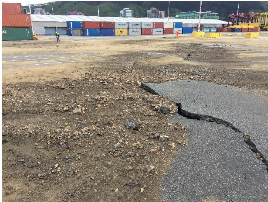
Figure 5.34: Widespread liquefaction of gravelly end-dumped quarry rock reclamation in container stacking area inland of Thorndon Wharf (S41.276608° E174.786309°, taken on 21NOV16)
