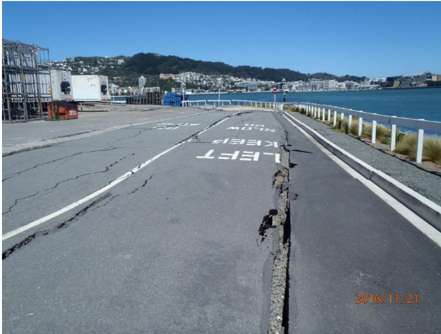
Figure 5.55: Ground cracks in area west of the CS building and along the southwestern slopes of CentrePort (looking south). The CS building can be partially seen on the upper left corner of the photograph. (S41.281478° E174.784430°, taken at 1418 hrs on 21NOV16)
