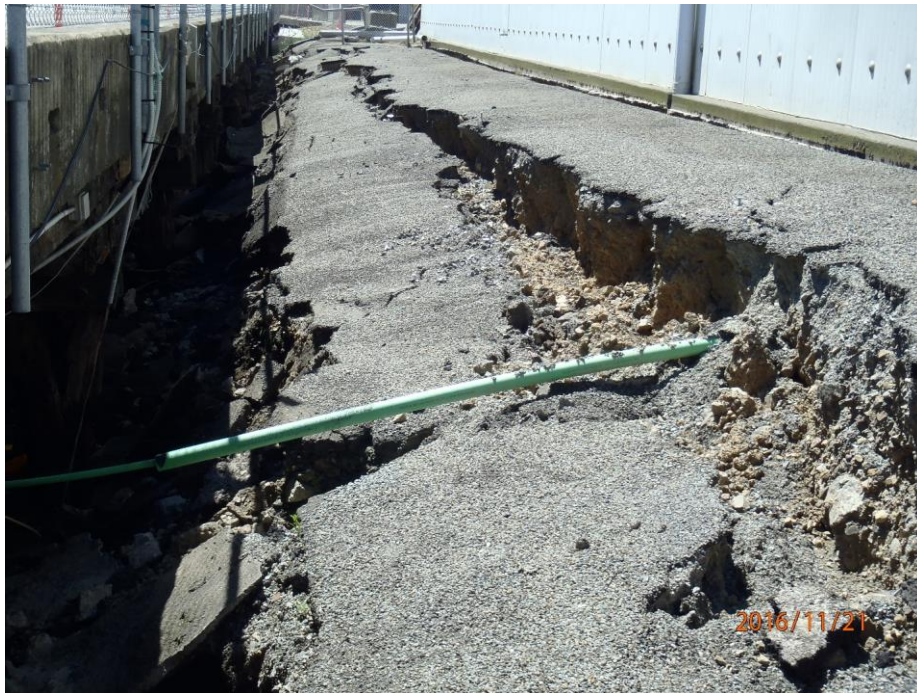
Figure 5.54: Looking north along the west wall of the CS building. The ground settled approximately 530 mm relative to the pile-supported bulkhead of King's Wharf, which is shown at the left side of the photograph. (S41.280923° E174.784389°, at 1411 hrs on 21NOV16)
